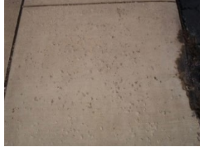
Figure 16: Very Good (8) - Minor defects caused by weathering. Still looks acceptable.
