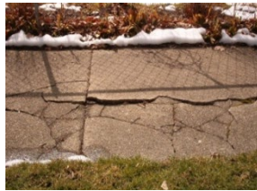
Figure 21: Poor (3) - Functionality is almost gone. Negative aesthetics.
