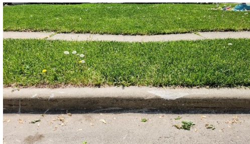
Figure 28: Example of utility service sinking
