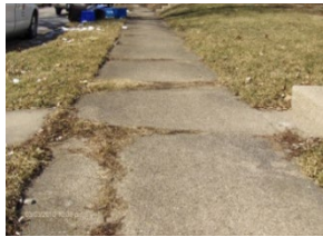
Figure 20: Fair - (4) - Still usable by most. Not easily navigated by runners, stroller users, and wheelchair users. Lacking aesthetic appeal.
