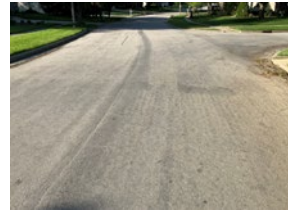
Figure 6: Good + (7) - First signs of aging. Some traffic wear with 1/4-inch surface cracks. No patching.
