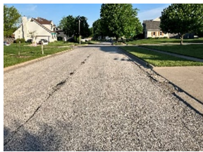
Figure 9: Fair - (4) - Significant aging. Patching in fair condition. Slight rutting.
