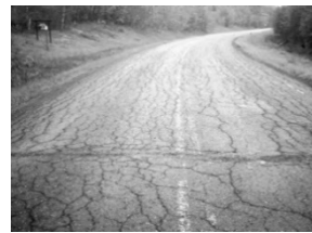
Figure 11: Very Poor (2) - Severe deterioration. Excessive patching in poor condition. Needs major rehabilitation or reconstruction.
