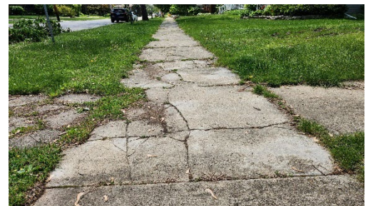
Figure 32: Example of old and broken sidewalk
