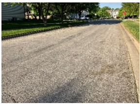
Figure 8: Fair + (5) - 1/2-inch open surface cracks. Surface aging. Some patching.
