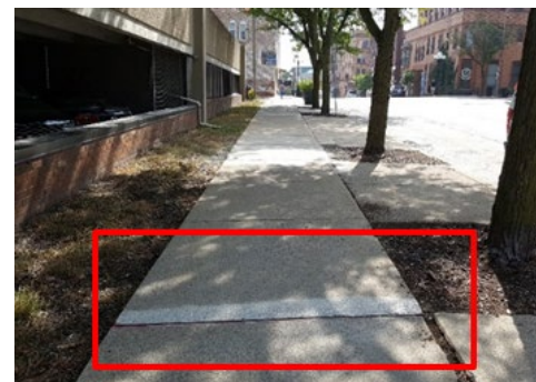
Figure 51: Sidewalk vertical displacement repaired using panel saw-cutting
