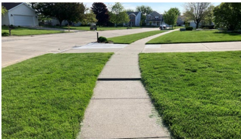
Figure 27: Example of settled panel
