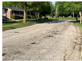
Figure 10: Poor (3) - Closely spaced surface cracking. Patches in fair to poor condition. Occasional potholes.
