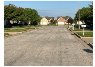
Figure 7: Good - (6) - Shows signs of aging. Occasional patching.
