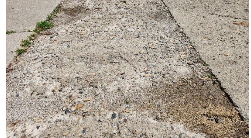
Figure 26: Example of spalled concrete
