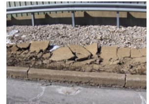
Figure 23: Failed (1) - Sidewalk is impassable. Needs to be replaced.
