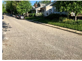
Figure 5: Very Good (8) - Minimal surface cracking.
