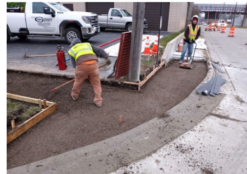
Figure 50: City contractors work to install sidewalk, curb, and gutter at an intersection
