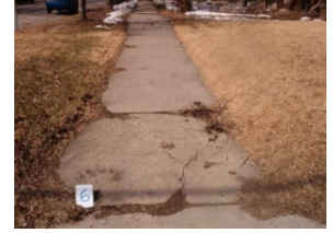
Figure 18: Good - (6) - Minor defects. Functionality and aesthetics are slightly lowered. Still acceptable.
