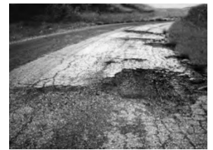
Figure 12: Failed (1) - Needs total reconstruction.
